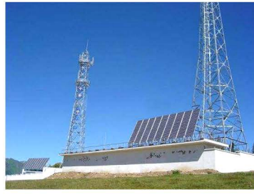
communication base station
